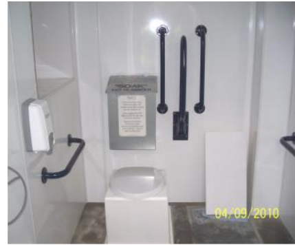
Components kit installed in a new Church extension in North Wales
