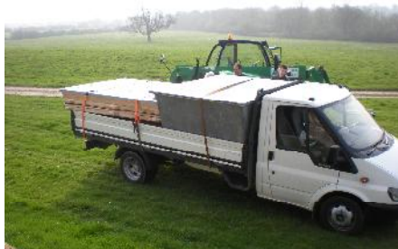
Delivery to site of the main components for a single toilet order.
